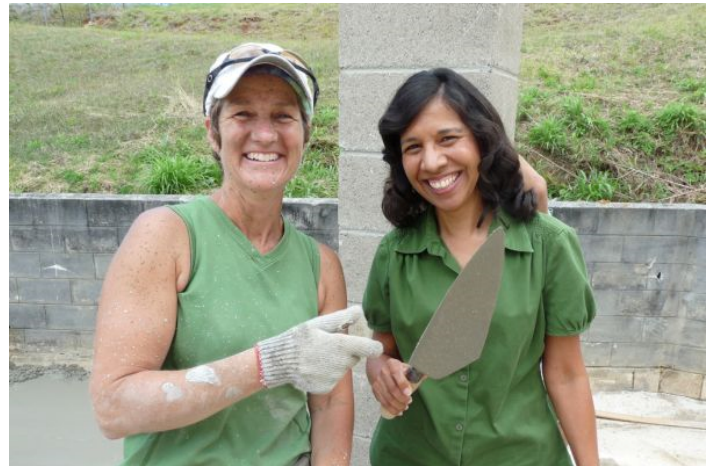
Figure 4: Jen Montour (left) and Eli Sabin (right) help pour cement on the Guam site in 2013.
