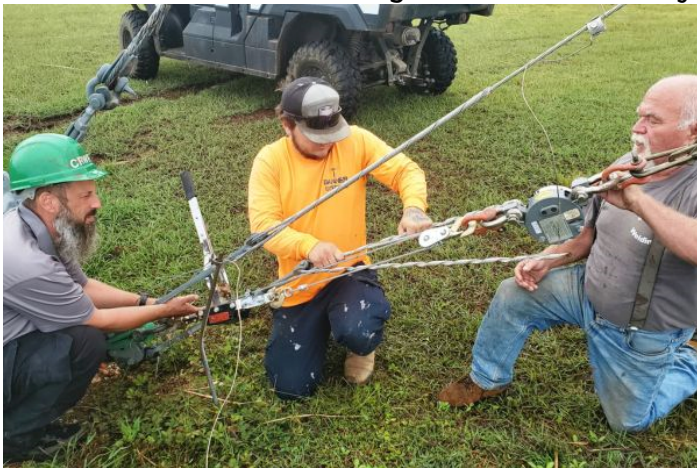
Figure 3: Members of TWR staff perform guy wire repair and maintenance following destruction to the Guam site by Typhoon Mawar in 2023
