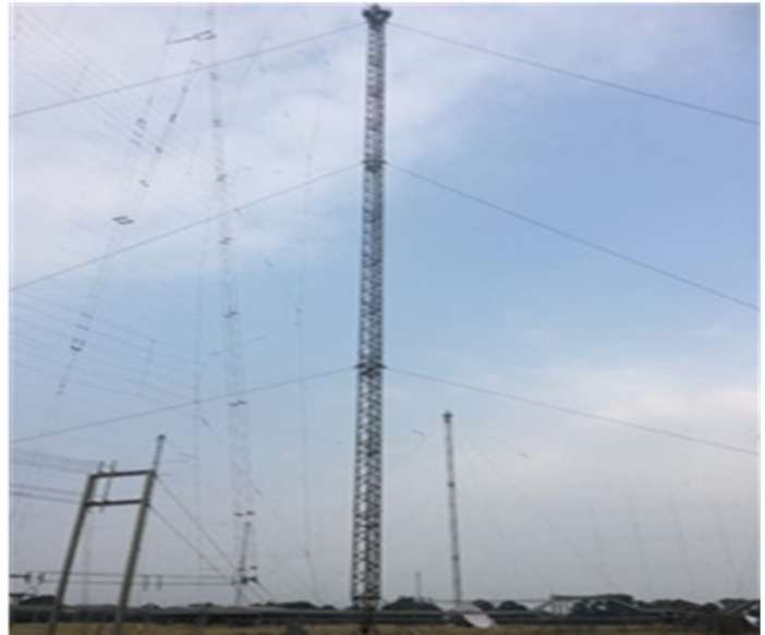
Non-radiating towers support the latticework of HF curtain antennas.
