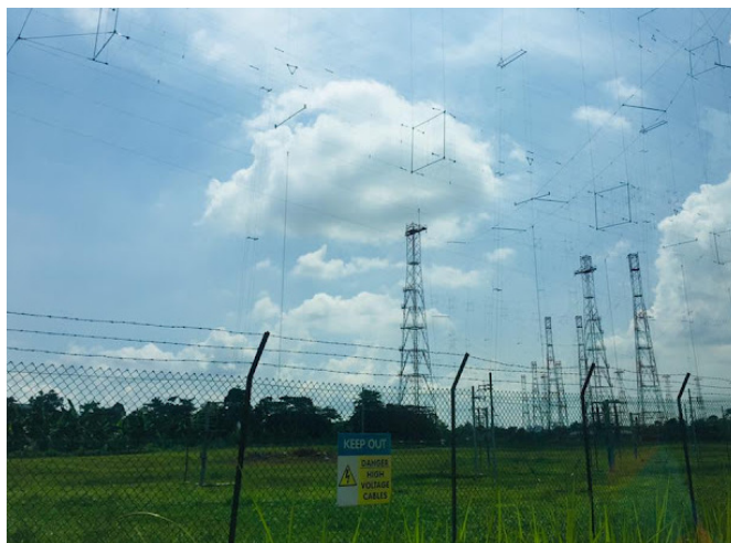
Antennas of BBC Relay Station, Kranji, Singapore
