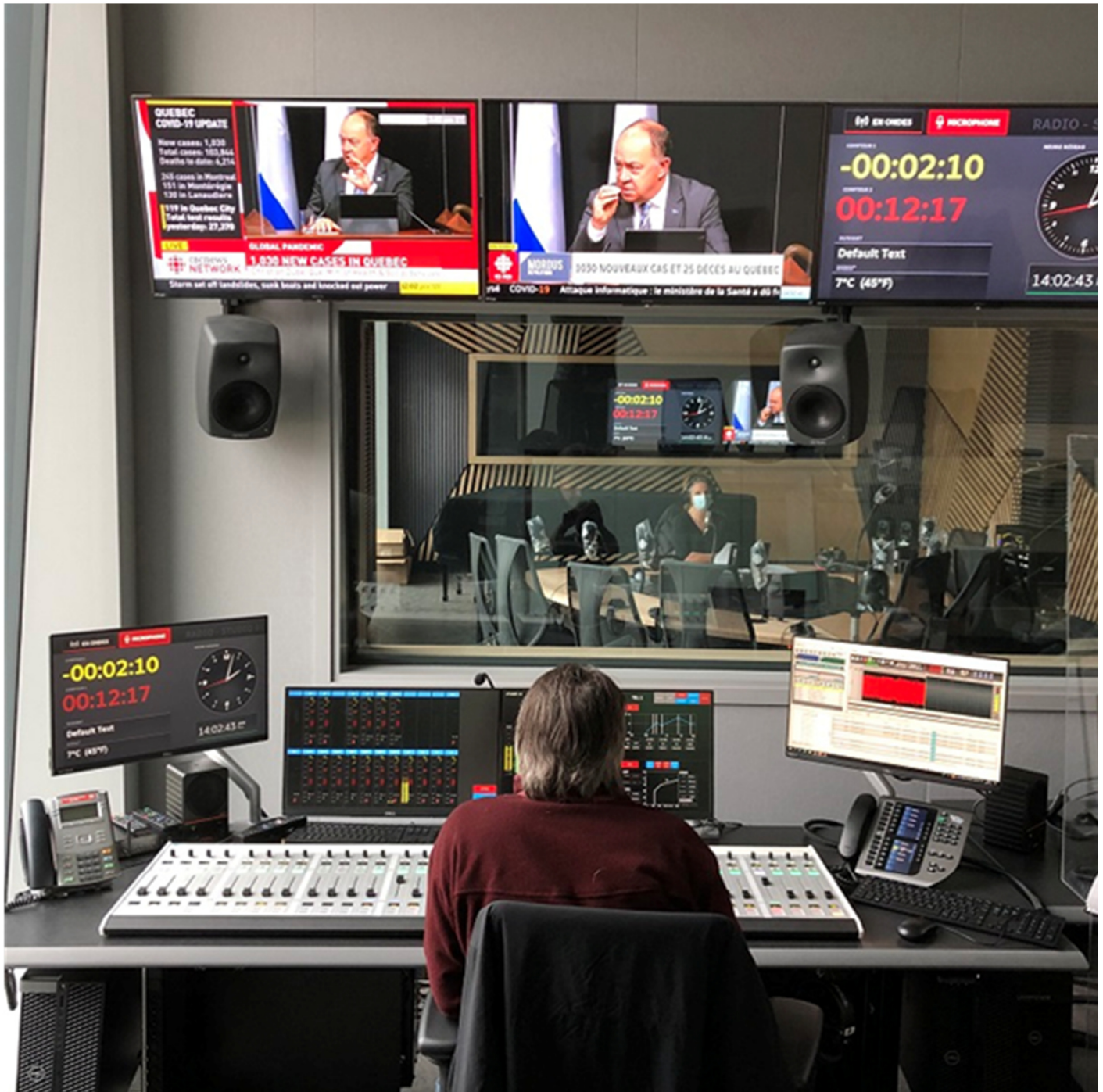
An audio technician at the desk of Studio 1, the facility’s biggest radio studio. The IDS display system is to the technician’s left and, above the window, the Lawo Ruby Surface, VisTool displays and Dalet playback. (Photos courtesy CBC/Radio-Canada)
