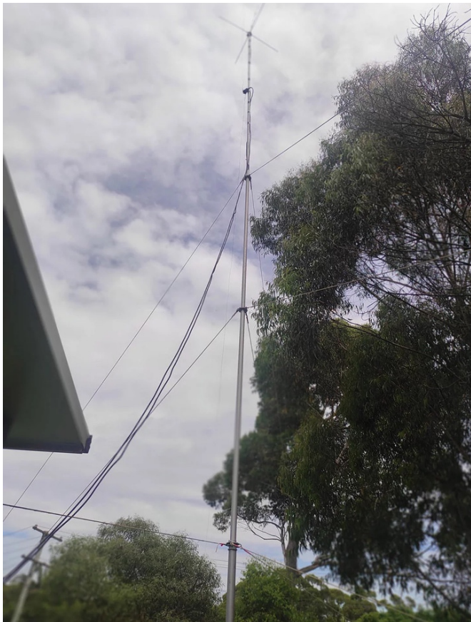
Island FM's shortwave and FM tower. The FM antenna is the very top of the tower and shortwave balun is mounted on the tower about halfway down with two thin wires coming out of it. [Photo courtesy of Island FM]
