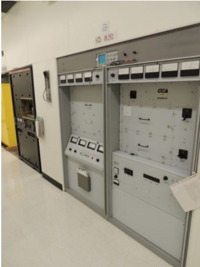
WWV 10MHz transmitter and standby
