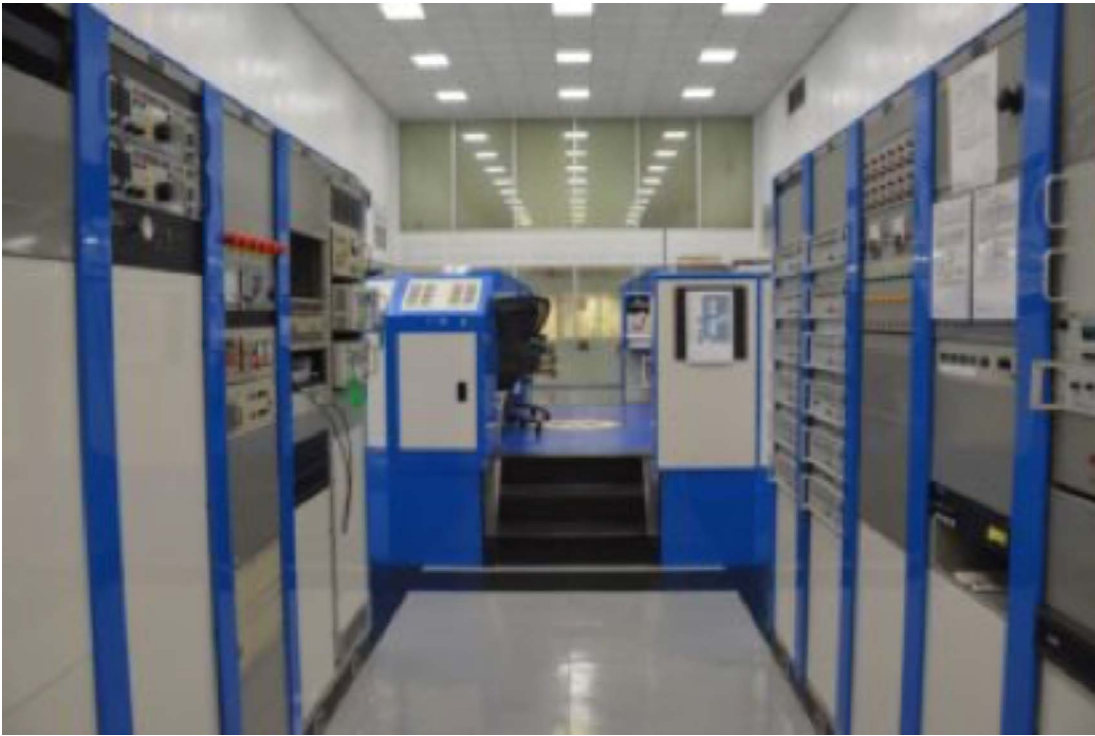
The Control Room in the U.S. government's Edward R. Murrow Transmitting Station near Greenville, North Carolina. Credit: Thomas Witherspoon.
