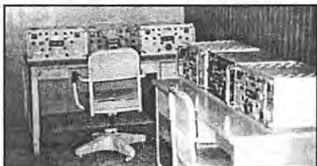
Collins receivers in a bunker under the Presidential Palace.
