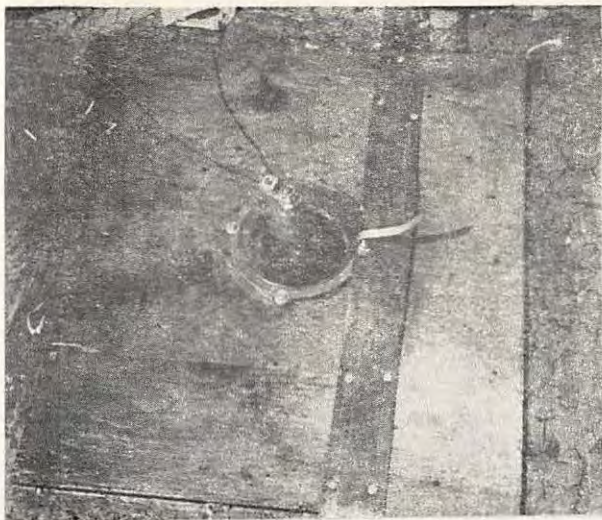
Antenna feed-thru on main deck. Arcing took place at this point, restricting power to 5-6 kw on 1160 kHz. Arcing problem was cured by going to centered inverted-V antenna (see October CB).
