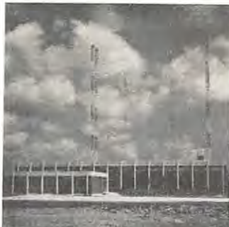
TWR'S TRANSMITTERS ON BONAIRE
